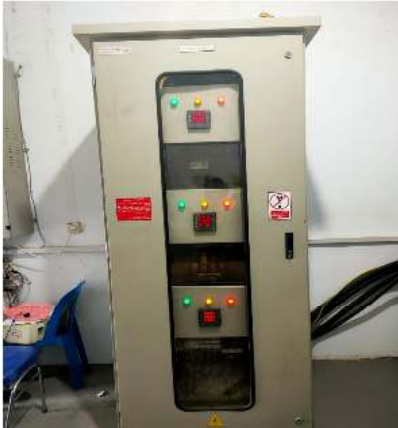
Gambar 3.4 Panel Box listrik reset
