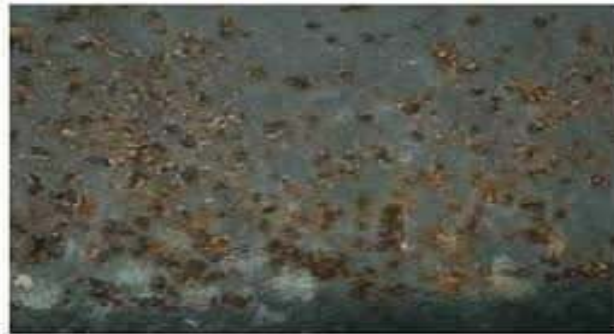
Gambar 2. 7 Korosi sumuran (Sumber : Jaya, dkk, 2010)
