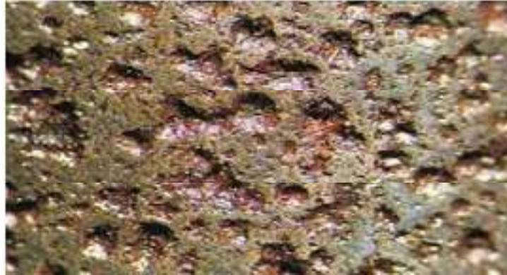
Gambar 2.5 Korosi sumuran (sumber : Jaya,dkk,2010)
