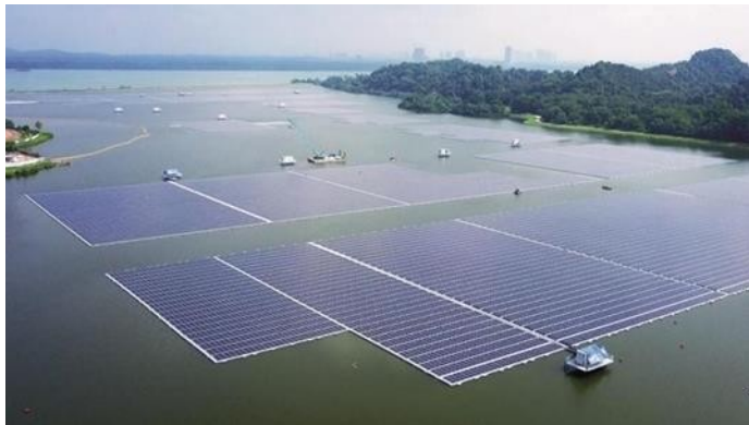
Gambar 3.8: PLTS Floating solar system (Sujay, 2017)
