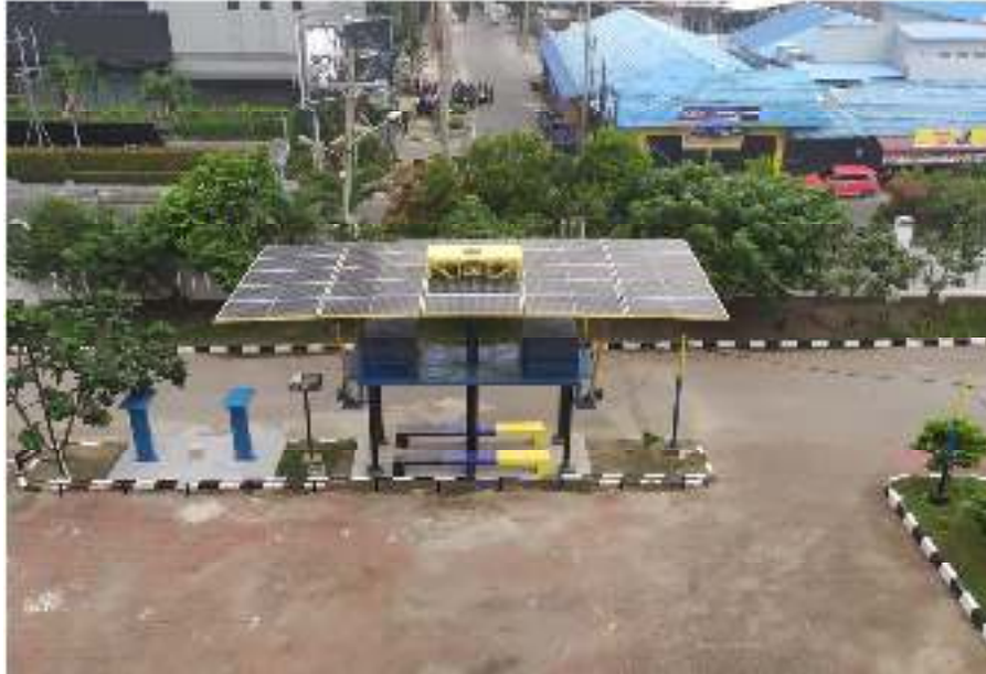
Gambar 3. 2. PLTS OFF GRID 10 kWp
