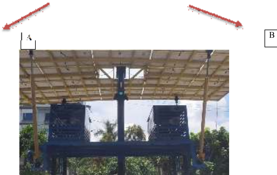
Gambar 3. 6. (A)Box Inverter 1, (B) Box Inverter 2
