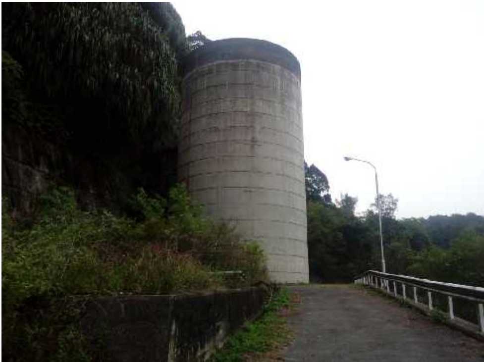
Gambar 3.5. Tangki Peredam/Surge Tank
