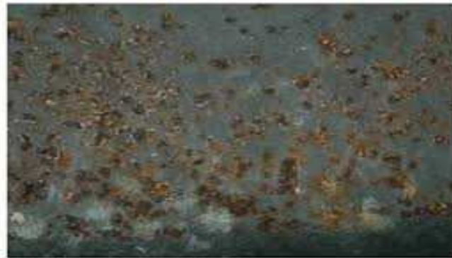
Gambar 2.6 Korosi sumuran (Sumber : Jaya, dkk, 2010)
