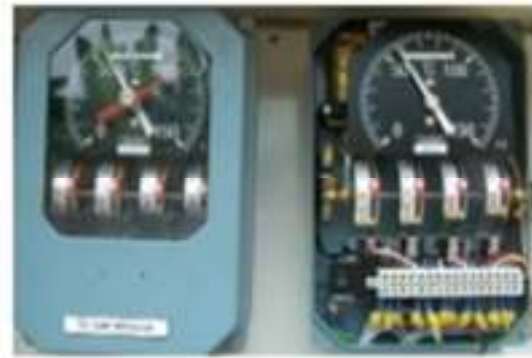
Gambar 2.5. Relay HV/ LV Winding Temperature
