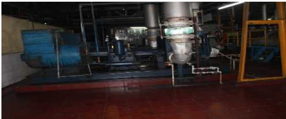
Figure 3.1 Electric induction motor generator driven steam turbine driven
